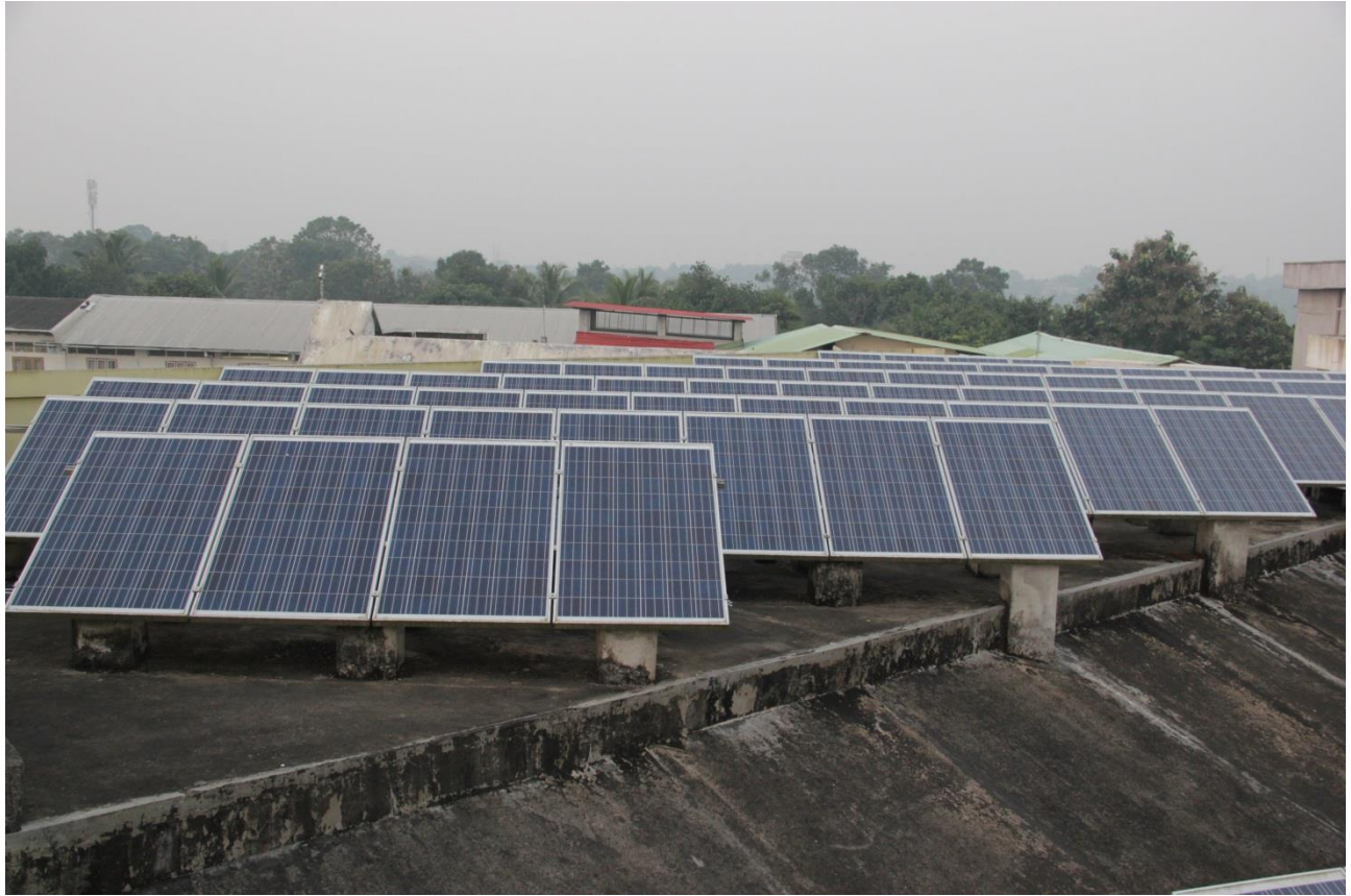
The Solar Panel installed at MACFAST Campus
